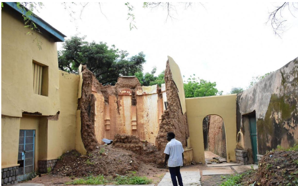
Figure 1: Collapsed roof of an earthen monument in the Nasarawa Palace
