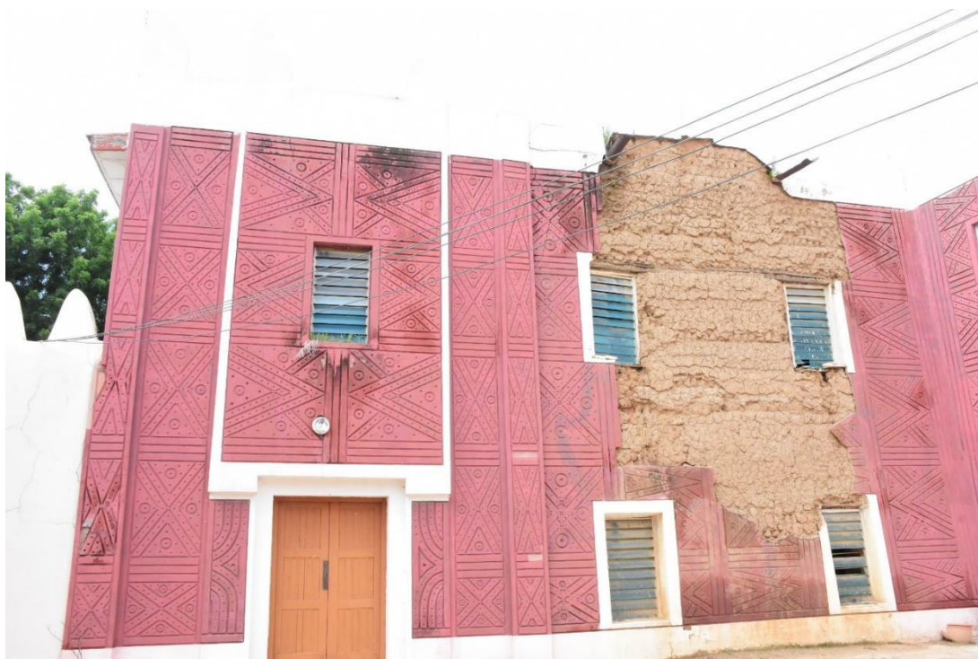
Figure 2: Collapsed cement plaster layer on earthen surface
